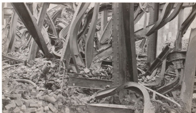
Image depicts bent steel after a building fire.
