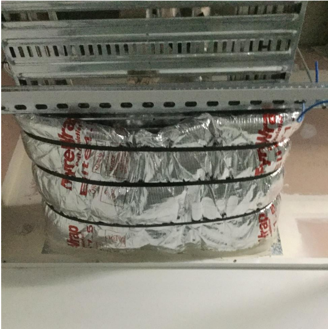
A final cable tray installation with a cable trays, multiple cables all nicely finished with EyreWRAP to provide a full FRL of -120/120 in this case
