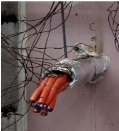
A small bundle of larger core power cables being fire tested without a cable tray; note the Trafalgar TWRAP insulation
