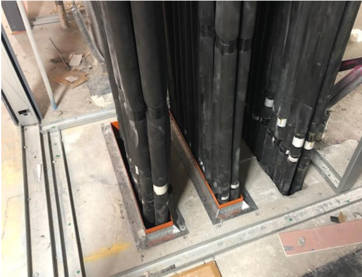
Trafalgar FyreBOX Maxi's being installed to protect large banks of the same service type (insulated copper services) passing through a fire rated floor slab
