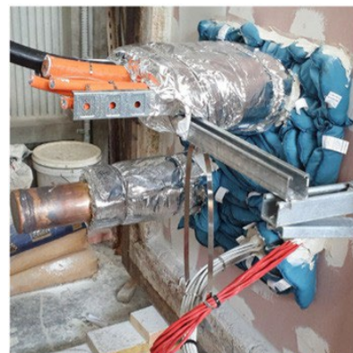
Image shows: Metal Pipes up to 100mm, unwrapped bundles of small cables and cable trays
