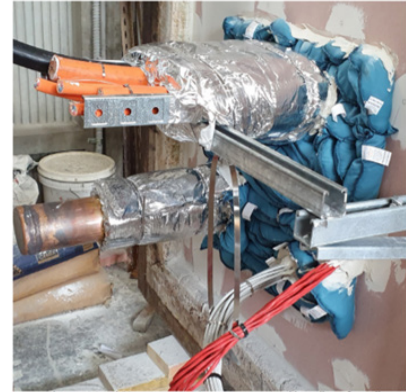
Image shows: Metal Pipes up to 100mm, unwrapped bundles of small cables and cable trays
