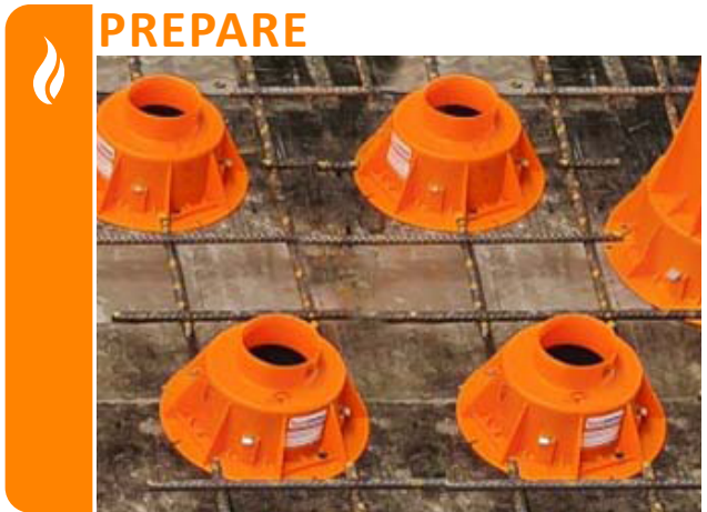
Fix the collar in place to the form work ensuring 50mm separation from edge to edge between each collar.
