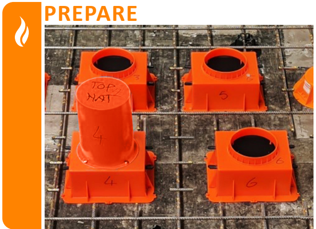
Fix the collar in place to the form work ensuring 50mm separation from edge to edge between each collar.
