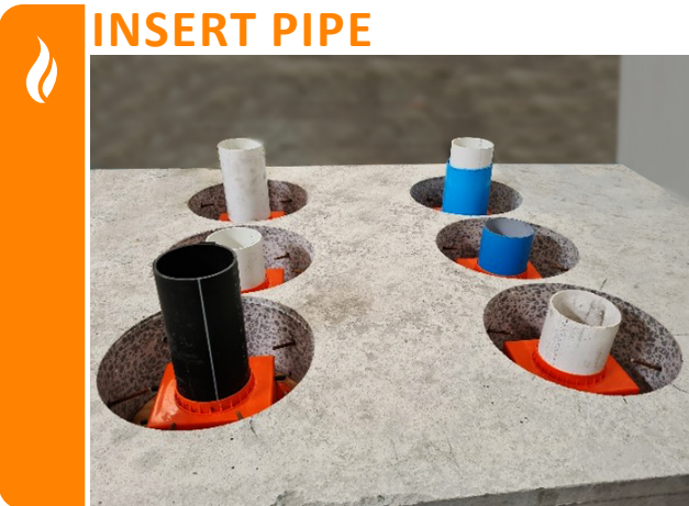
To ensure concrete does not fill into the collars, install a pipe former to the collar.
