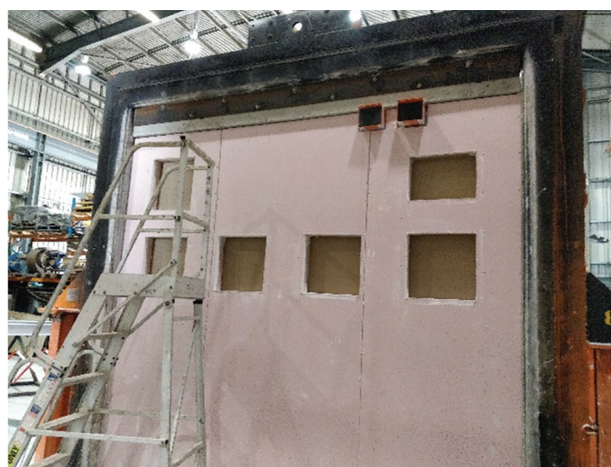
Installation of a full size fire rated plasterboard wall for a fire resistance test to AS1530.4 (with access panels)
